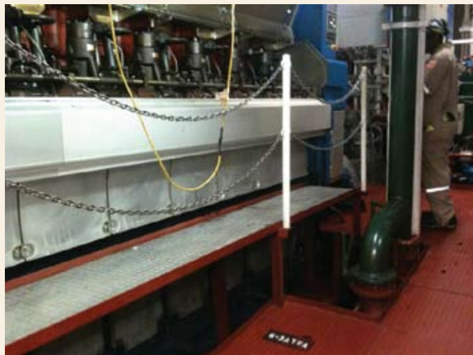
Inboard Starboard Engine showing raised working platform and safety stanchions and chains
